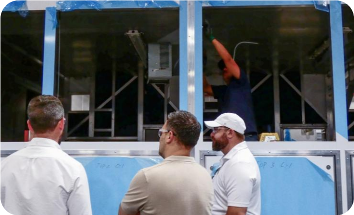
Backup generation inspections for Moses Lake
