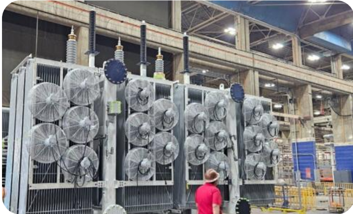
Transformer delivery in Sharon, PA
