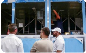
Backup generation inspections for Moses Lake
