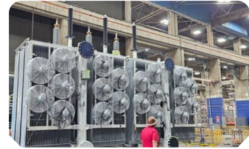
Transformer delivery in Sharon, PA
